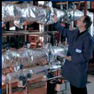
Ready assembled control systems
